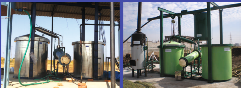
Field Level Distillation Plant ( SS & MS )
