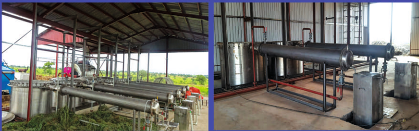
100 & 50 TPD Steam Distillation Plant
