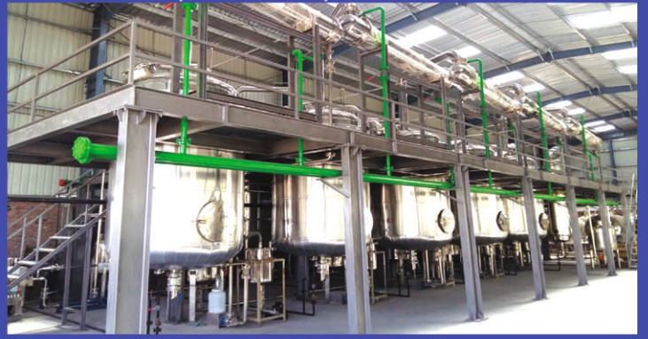
Turmeric (Curcumin) Extraction Plant
